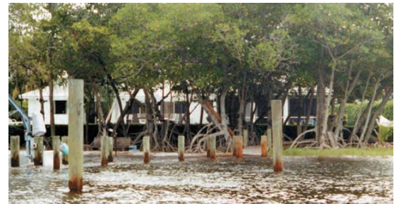
Undercutting with red mangrove
